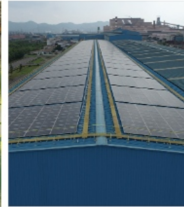
Initiative towards Carbon Neutral with installation of Solar PV 1.2 MWP at Hot Rolling Plant
